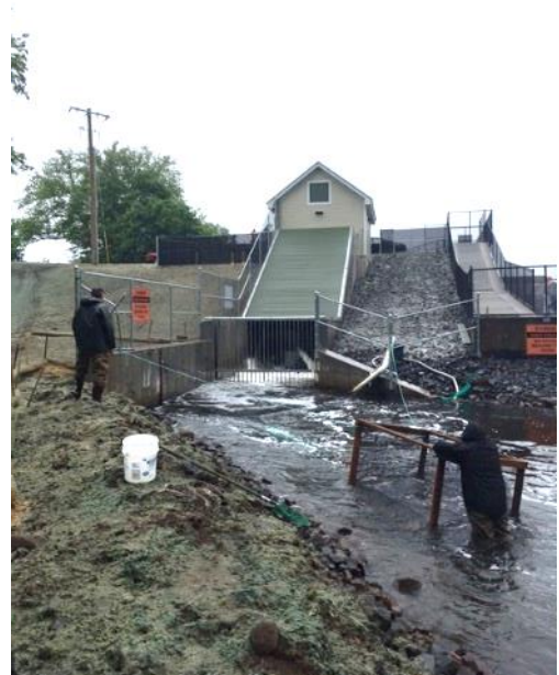
The Archimedes Screw is under the green cover below the powerhouse. The Hanover Pond Denil Fishways is to the far right. In this photo, Fisheries Division staff position a mesh trap and a net to capture shad coming down the Screw.
